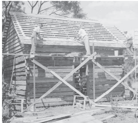
The Sanders Cabin in 1958 during reconstruction on the Shaw House grounds. Heading up the project is Roy Newton (center).
