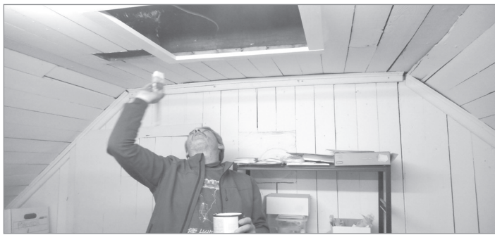
What happens when there is no heat or cooling in the Shaw House second floor? Well, one opens up the attic to find squirrels have eaten through the ductwork. Special thanks to Wayne Almas who created entrances for the HVAC folks to help fix the problem.
