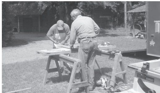
Workers cut planks to replace old rotten ones at the historic Shaw House. They also repaired parts of the Sanders Cabin. More repairs are still needed to the back part of the cabin, that is below grade and susceptible to rot from water damage and a magnet for termites.
