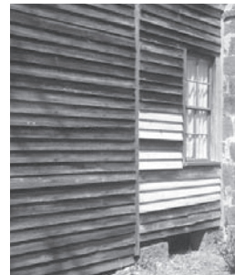
New strong boards are now in place in several areas of the Shaw House replacing the rotten and termite-infested parts.
