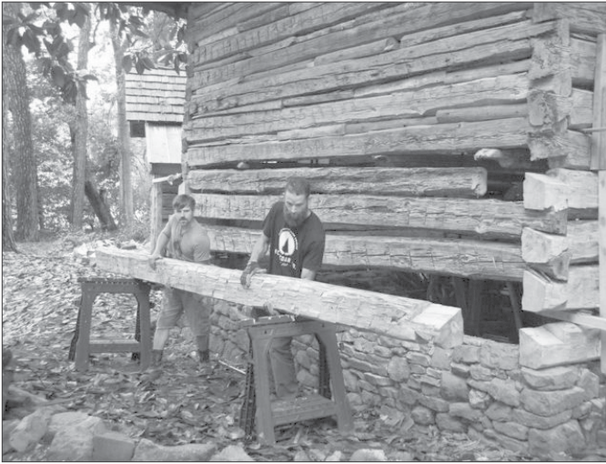
Josh Smith and Thad Lawrence restoring the Shaw House Tobacco Barn. Photo credit, The Pilot Newspaper .
